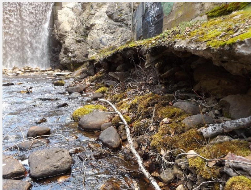
Evidence of Creek Downgrading Below Penticton Dam #2
