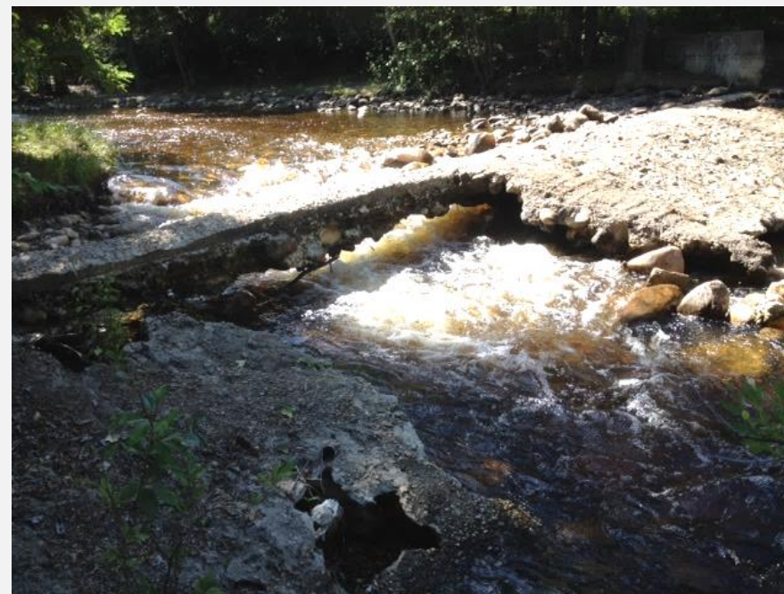
A failed concrete structure in Reach 9
