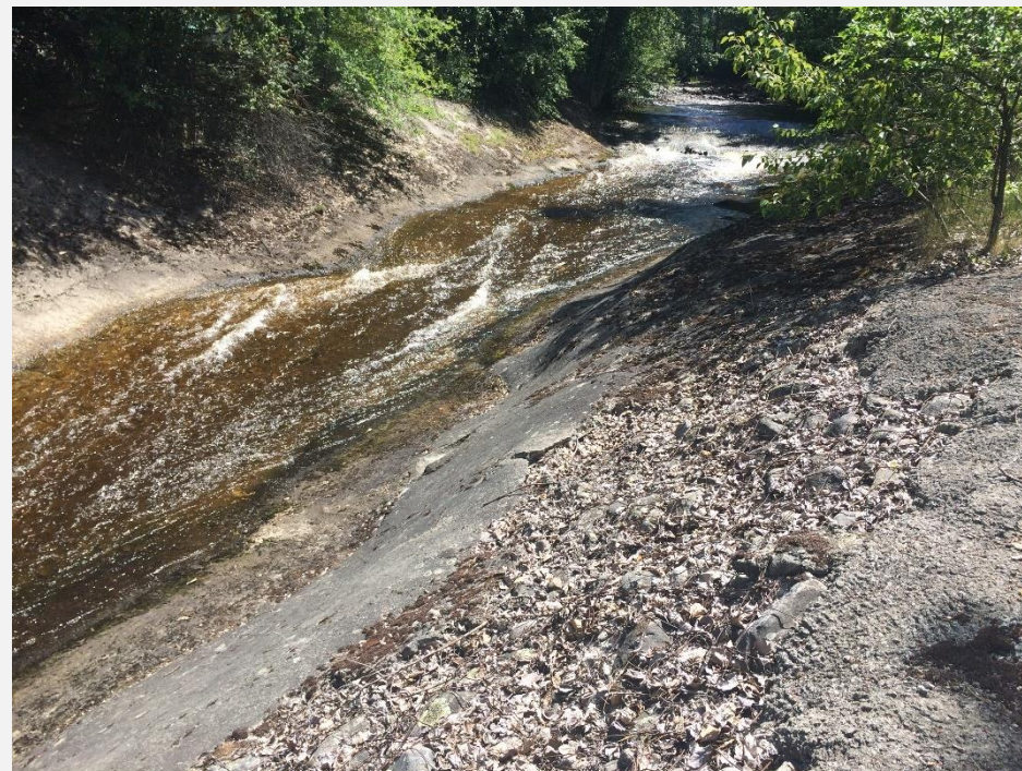
A concrete lining hole with visible mesh
