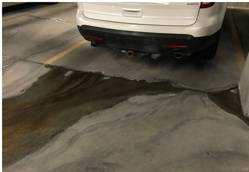
Figure 11. Water Seepage in a Parking Garage
