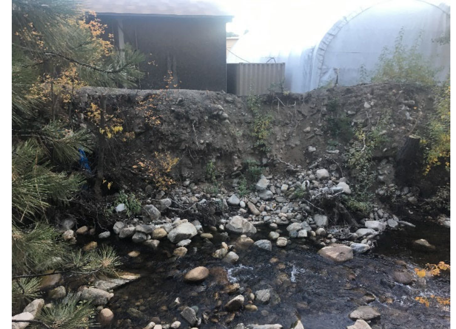
Unstable Ellis Creek Bank
