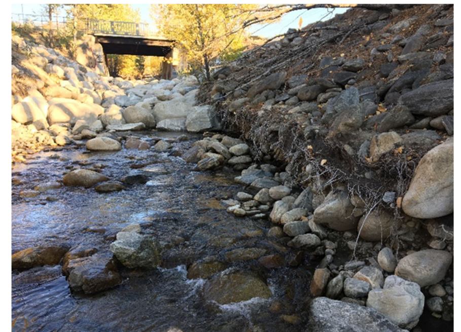
Degradation in Ellis Creek Channel (Dartmouth Road Bridge)
