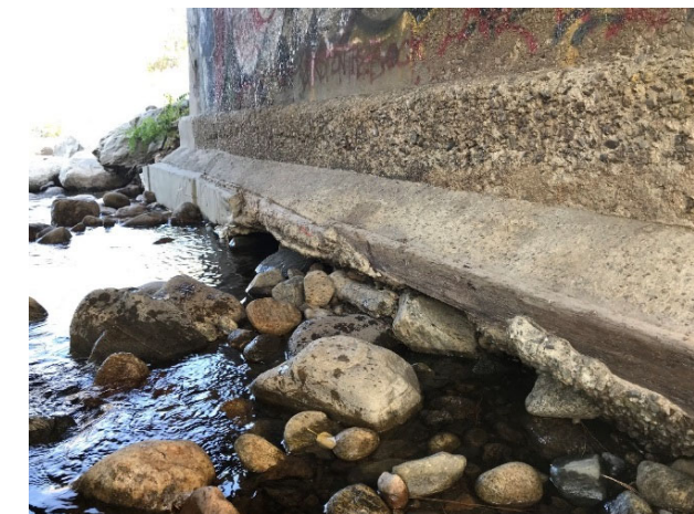
Channel Erosion at Dartmouth Road Bridge
