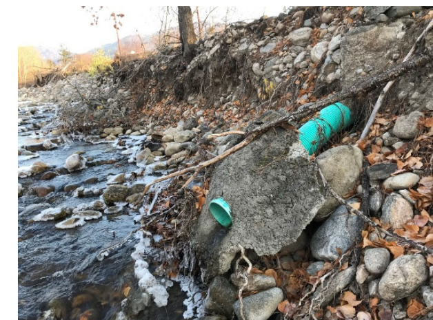
Dislodged Stormwater Outfall
