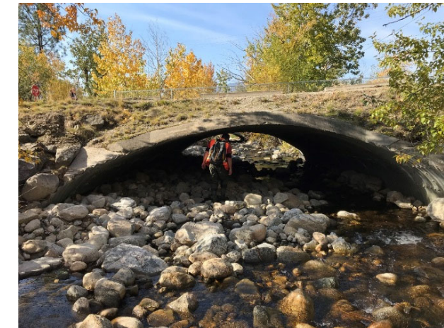
Deposition at East Hospital Access Bridge
