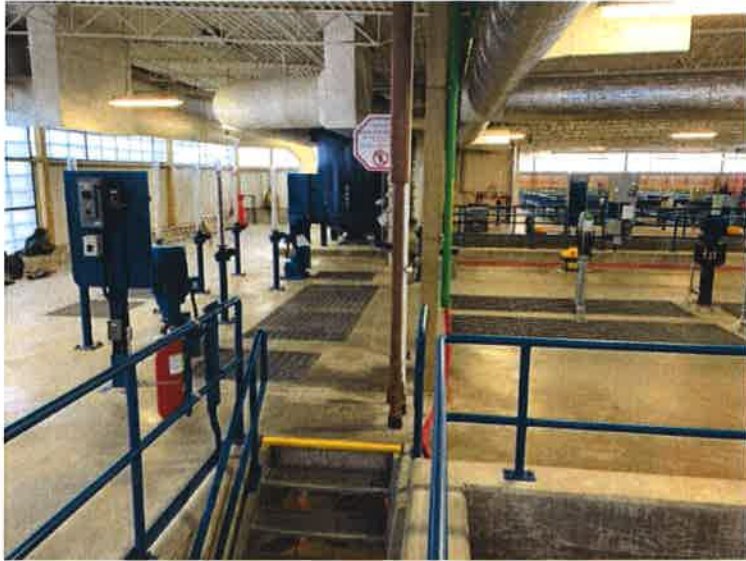
Figure 5: Water Treatment Plant Blend Chamber
