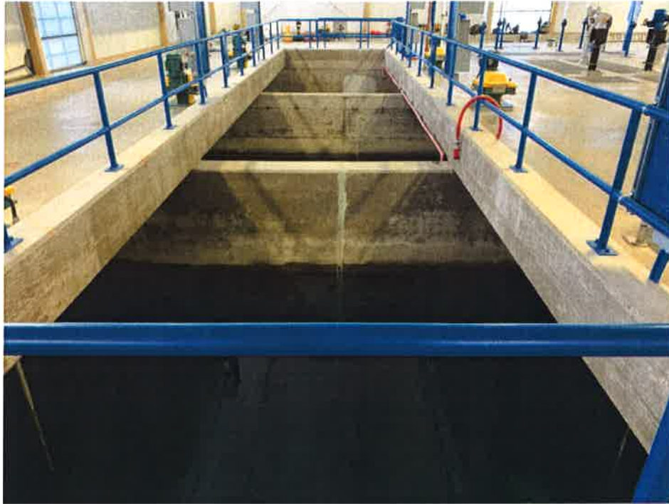
Figure 6: Flocculation Tank Mixers
