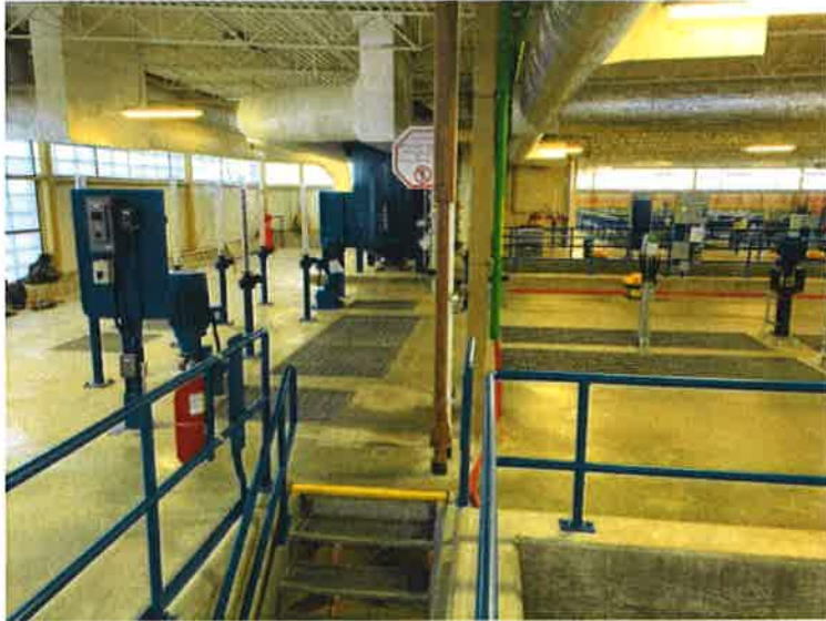
Figure 5: Water Treatment Plant Blend Chamber
