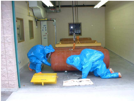
Changing Chemical Tanks
