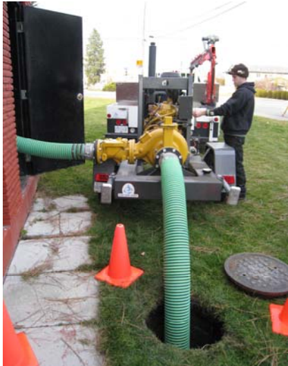
Lee Ave By-Pass Pump
