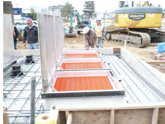
Lee Avenue Lift Station
