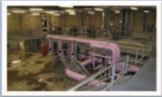
New reclaimed water pumping station and new UV disinfection system
