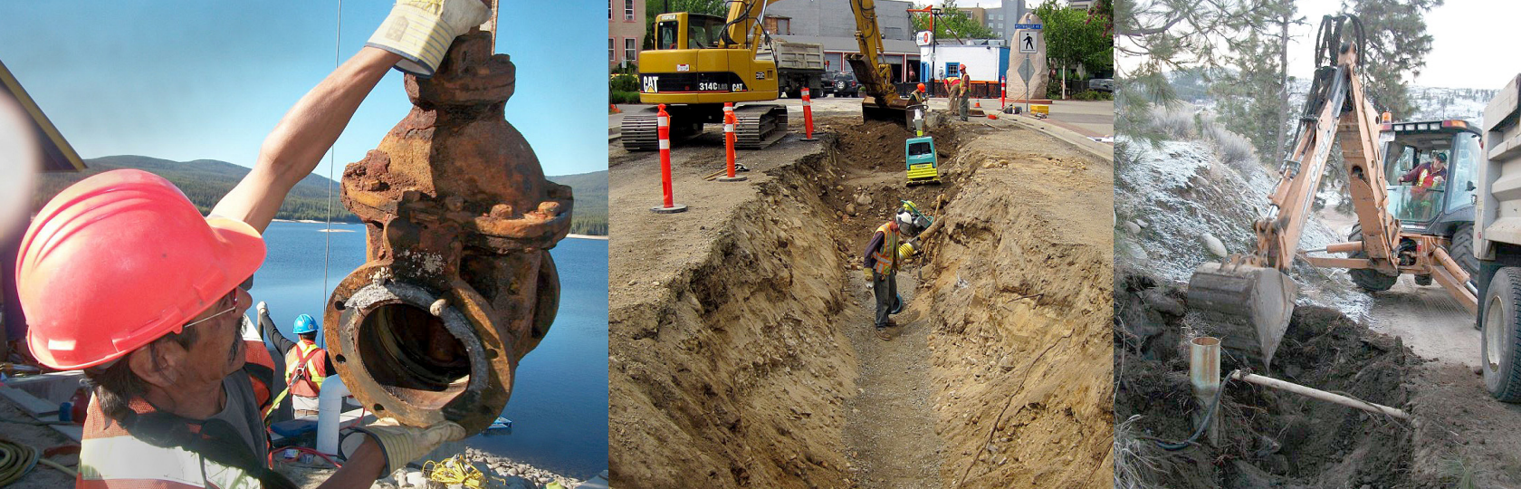
Engineering and Public Works staff were involved in a variety of projects this year, conducting creek repair, dam upgrades and underground infrastructure replacement, in addition to planning the 2013 projects to come.
