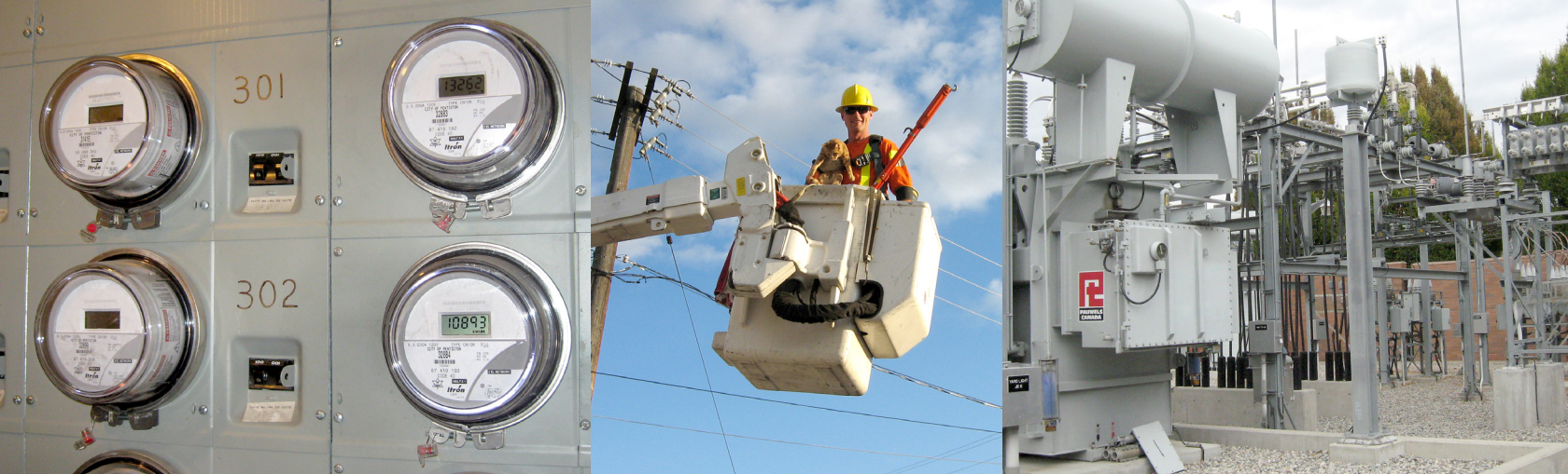
The Electric Utility handles all City electrical infrastructure and equipment, large and small. Staff responded to a variety of customers needs, including coming to the aid of a neighbourhood cat who ventured too far up a power pole (above centre), proving that no call is too small.
