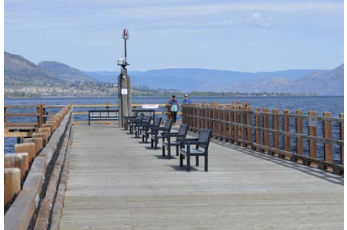
Council approved repairs to the Kiwanis Pier to reverse damage sustained during a high-water event in 2017 leading to its closure for the remainder of 2017 through fall 2018.
